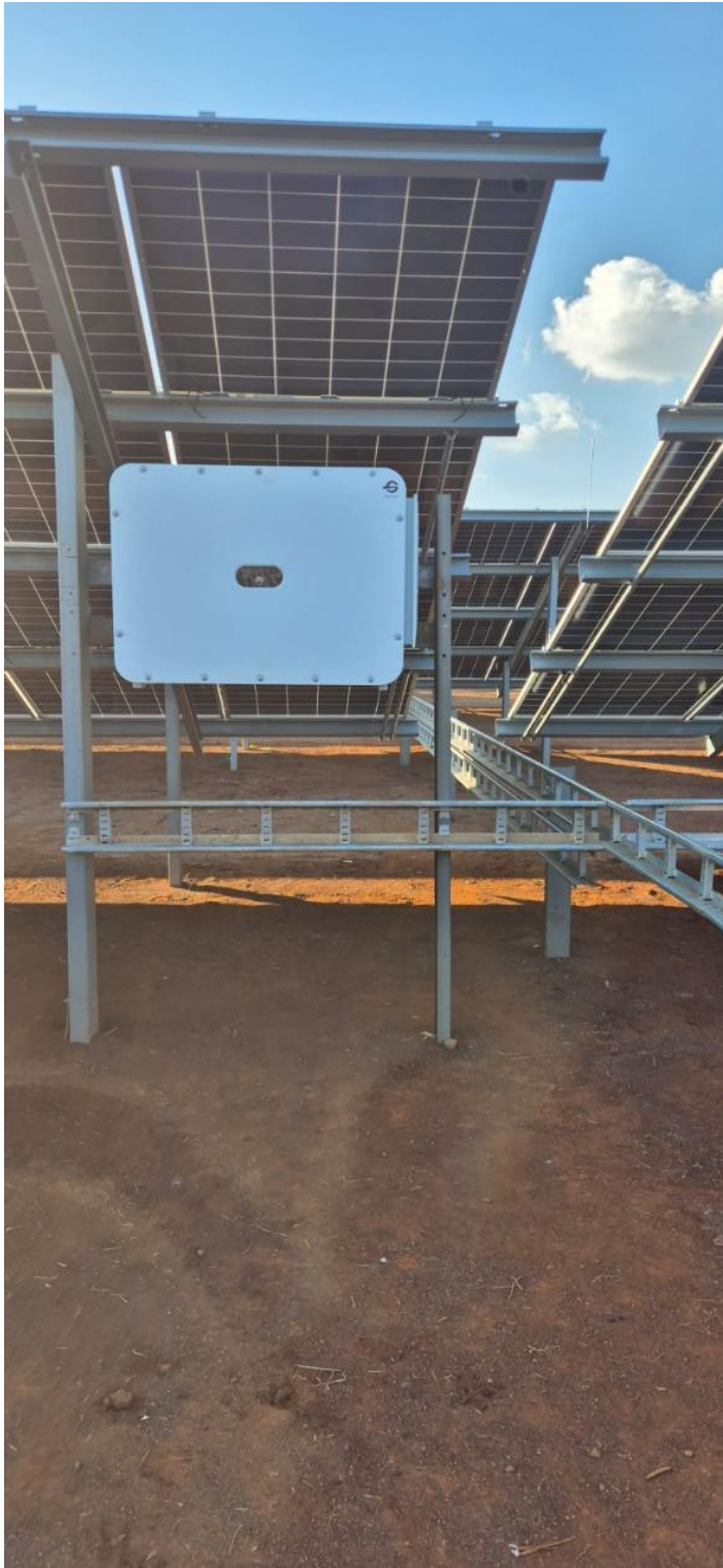
A maximum gap of 1000 mm between tables, with cable racks installed in some instances.
